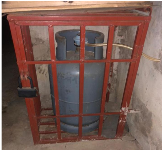
Figure 10: Right way of Storing a Cylinder at Home
