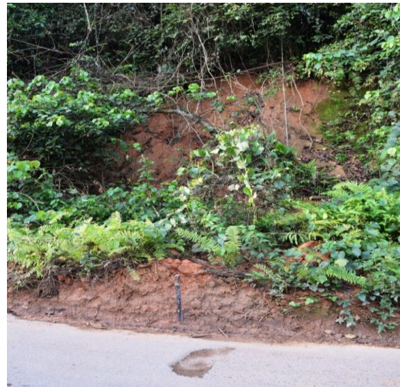
Figure 6b: Landslides of Bafut Forest
