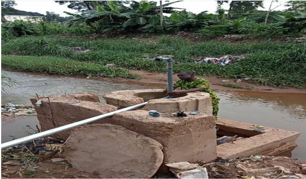
Plate 1. Sump/ Infiltration Structure
