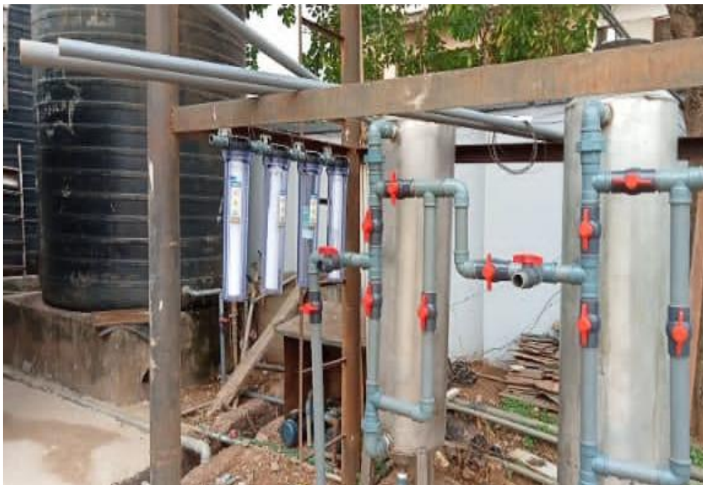
Plate 2. Local Water Treatment Plant
