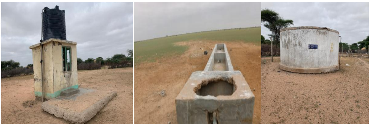
Plate 2 An old Water Kiosk, Water Trough and Storage Facility in Goreale Ward (Field Work, 2020)
