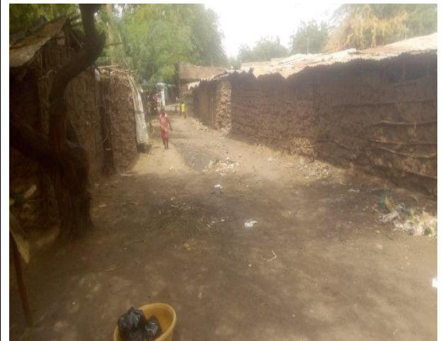
Plate 1: Low Quality House Made of Mud in Mororo Sub-Location. Source Field Data, (2022)
