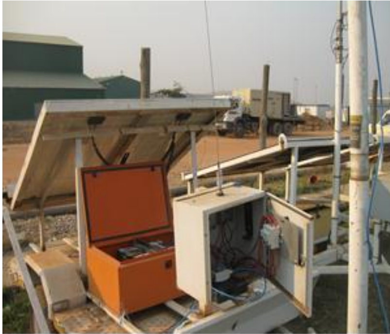
Figure 6: An integrated system of the VHF Motorola 2-way radio and Ubiquiti wifi bullet radio.
