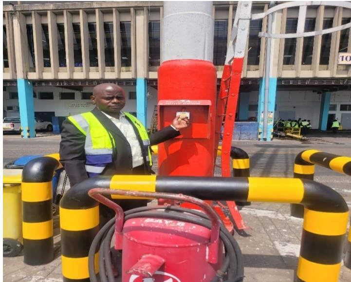
Photograph 1: Emergency Shut Down (ESD) at JKIA Bay No. 10
